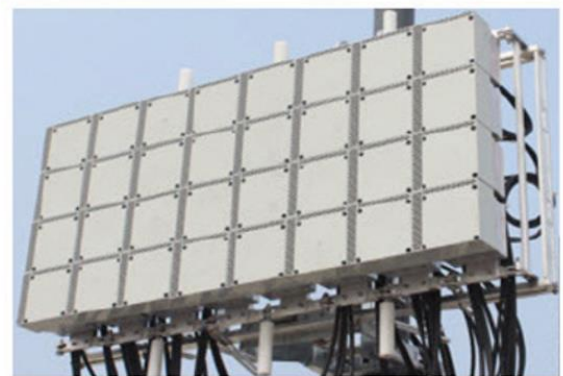
A massive MIMO antenna array for a Huawei 5G field trial.
